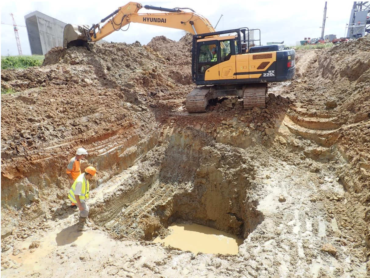
Fig. S1. Trench KOU-AR6-01, with giant exhaust-aimed and gantry infrastructures for Ariane 6 in the background (top left and right, respectively). Water fills the bottom of the stratigraphic sequence, thus covering the basal oyster-rich conglomerate and grey clays, being sampled by the excavator bucket. Photograph by A.H.
