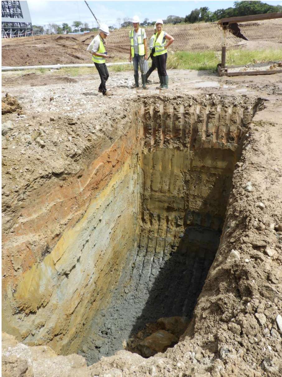
Fig. S5. Trench KOU-AR6-05, with the Ariane 6 rocket gantry in the background (left). The complete stratigraphic sequence is visible, starting by the basal oyster-rich conglomerate and grey clays. Photograph by P.-O.A.
