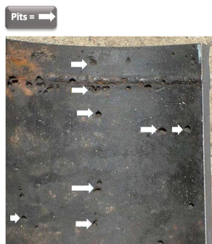
Figure 9. Pitting corrosion, photo of a section of an X65 steel pipe from an oil field in Western Australia.
